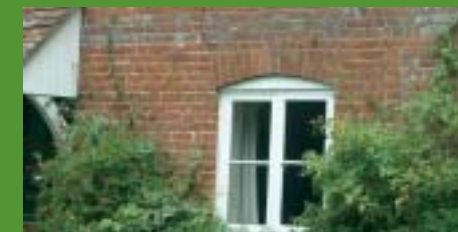
Arched windows and decorative brick with a plain clay tile porch are typical features.
